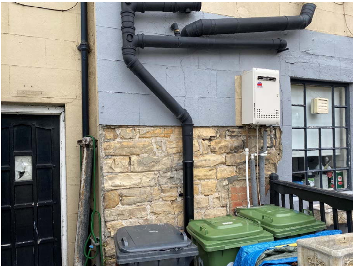
Exposed stonework below poor quality etched cement based render (existing southwest elevation)
