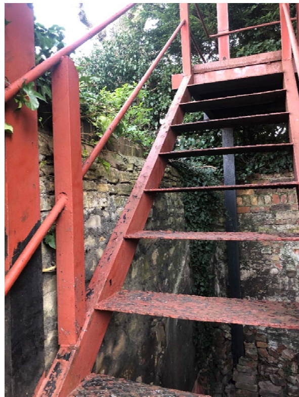
Existing stair sits on structure independent to party walls – the intention of new stair will follow the same principles.
